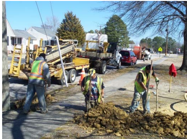
Construction crew members fill a trench after completing the boring work to install underground conduit at Lakeview.
